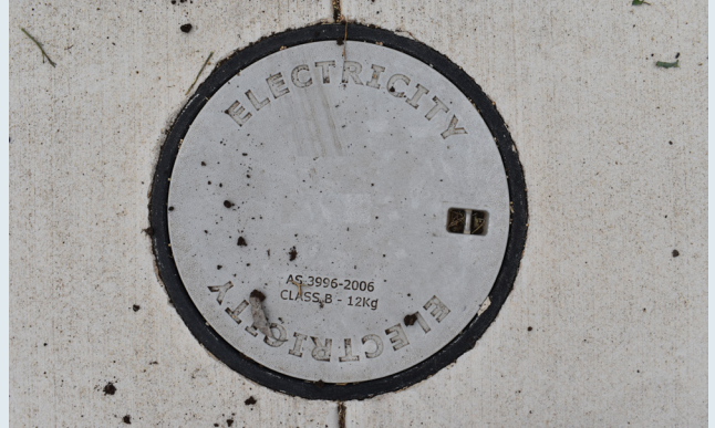
Figure 6: A pit indicating electrical cables below ground.
