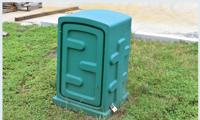
Figure 10: An underground connection pillar for an electrical installation on private property.
