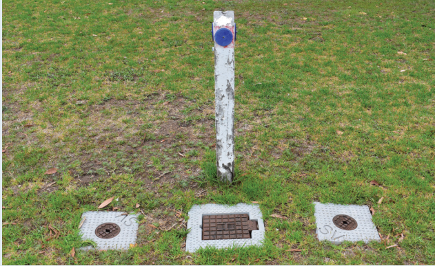
Figure 15: Hydrant connection points and water stop valves indicating water services underneath in close proximity.
