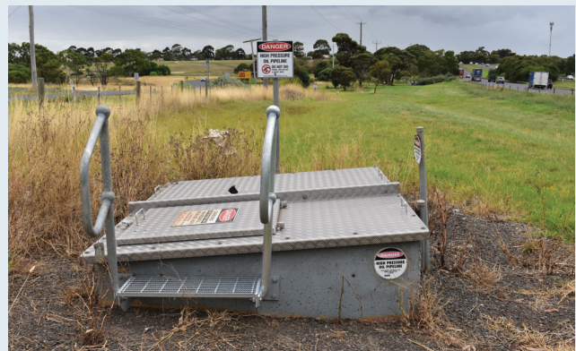
Figure 14: A warning sign and an access pit for underground high pressure oil pipeline.
