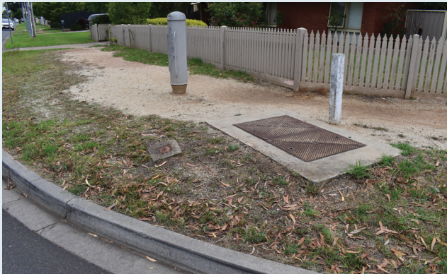
Figure 17: A telecommunication riser and pit indicating the presence of telecommunication cables in vicinity.
