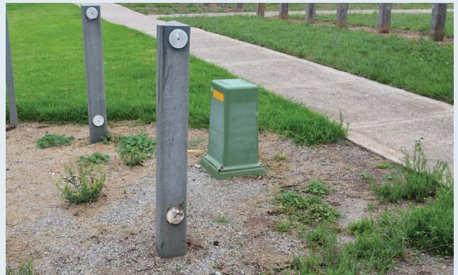
Figure 8: An underground pillar indicating low voltage electrical underground cables owned by the power company installed on public land.
